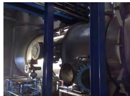
VALVE MOUNTED ON PLANT
